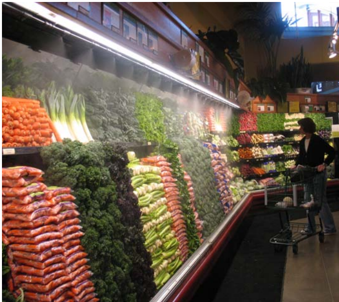
Corrigan systems for produce misting (UltraMist) and service case humidity (VaporPlus) have received NSF Certification.
